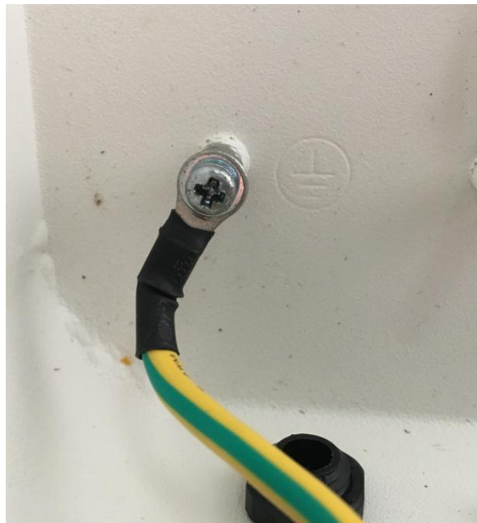
Figure 10. Internal Earthing Terminal
